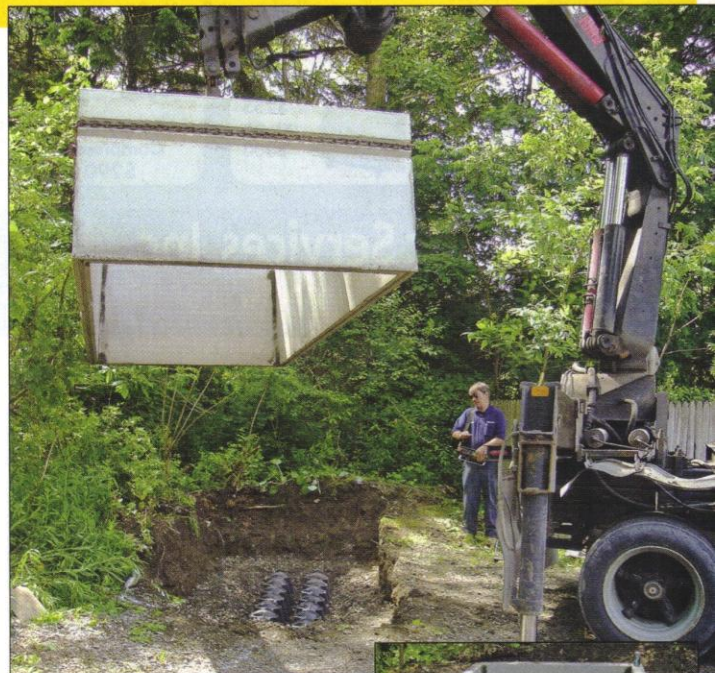
A mobile crane operator sets the low-profile, 1,000-gallon bottomless concrete tank over the two rows of Infiltrator chambers to form the odor-recovery bed. (Photos courtesy of Eric E. Murdock, P.E.)
