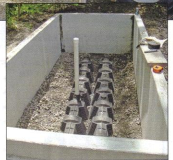
The odor-recovery bed is ready to be covered with organic-rich mulch. The vertical pipe is an observation port for evaluating air flow.
