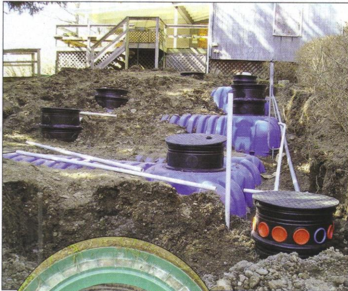
Above, five polyethylene tanks from Fralo Plastech are positioned end-to-end in a tight configuration. At left, the recirculation valve in the dosing tank returns 100 percent of the effluent to that tank if the water in it is low. If the liquid level in the dosing tank is high, 50 percent returns to that tank and 50 percent flows through a distribution box to the trenches and dry wells.
