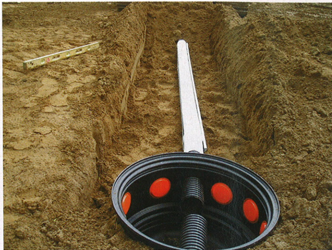
A sample collection point is installed for drip irrigation effluent. The perforated piping is 12 inches below the drip tubing.
