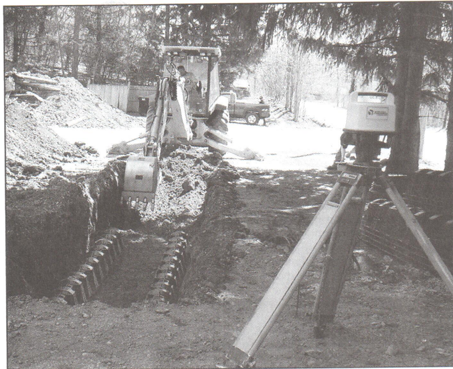
Foundation for alternative septic systems. They are essentially personal wastewater treatment systems for homes or businesses that treat the intake inside a tank before clear water is discharged back to the surface.
