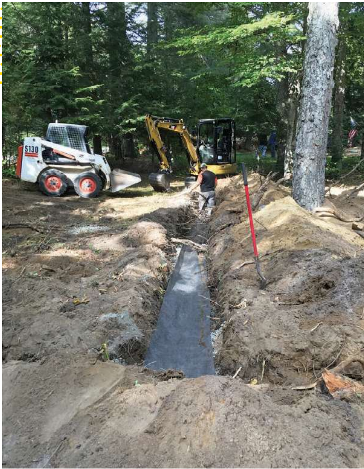
▲ A worker lays geotextile fabric over a 24-inch-wide stone-and-pipe trench. Equipment being used is a Caterpillar 304E2 CR mini excavator and Bobcat S130 skid-steer.
