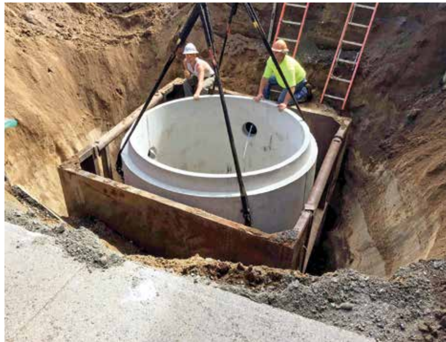
▼ Danny Stone (left) and Barry Cook from TJ Fiacco Construction help guide a riser onto the manhole base.
