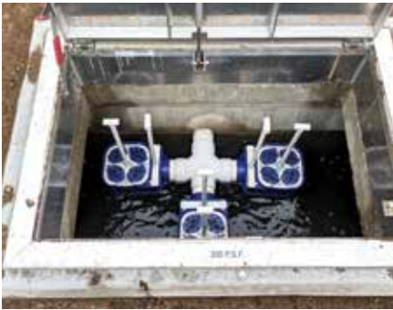
▲ Closeup of WW4 effluent filters from Clarus Environmental.
